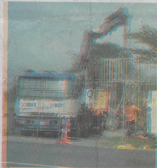
Electro Services Ltd services workers lift the height of a BDC pump station in north Derby Street above the one-in-100-year flood level. Photo: Lee Scanlon
