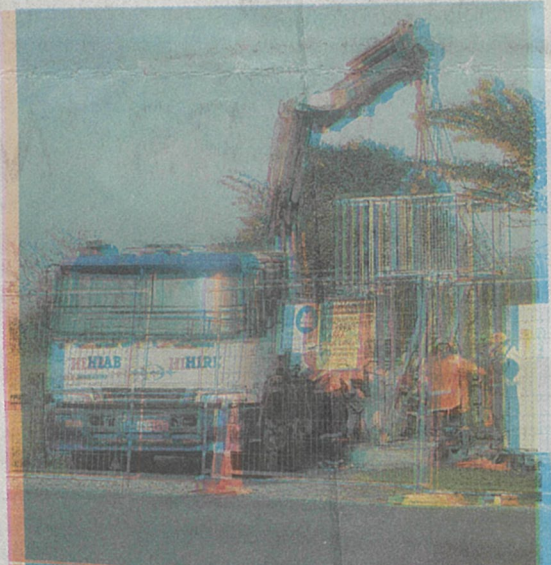
Electro Services Ltd services workers lift the height of a BDC pump station in north Derby Street above the one-in-100-year flood level. Photo: Lee Scanlon
