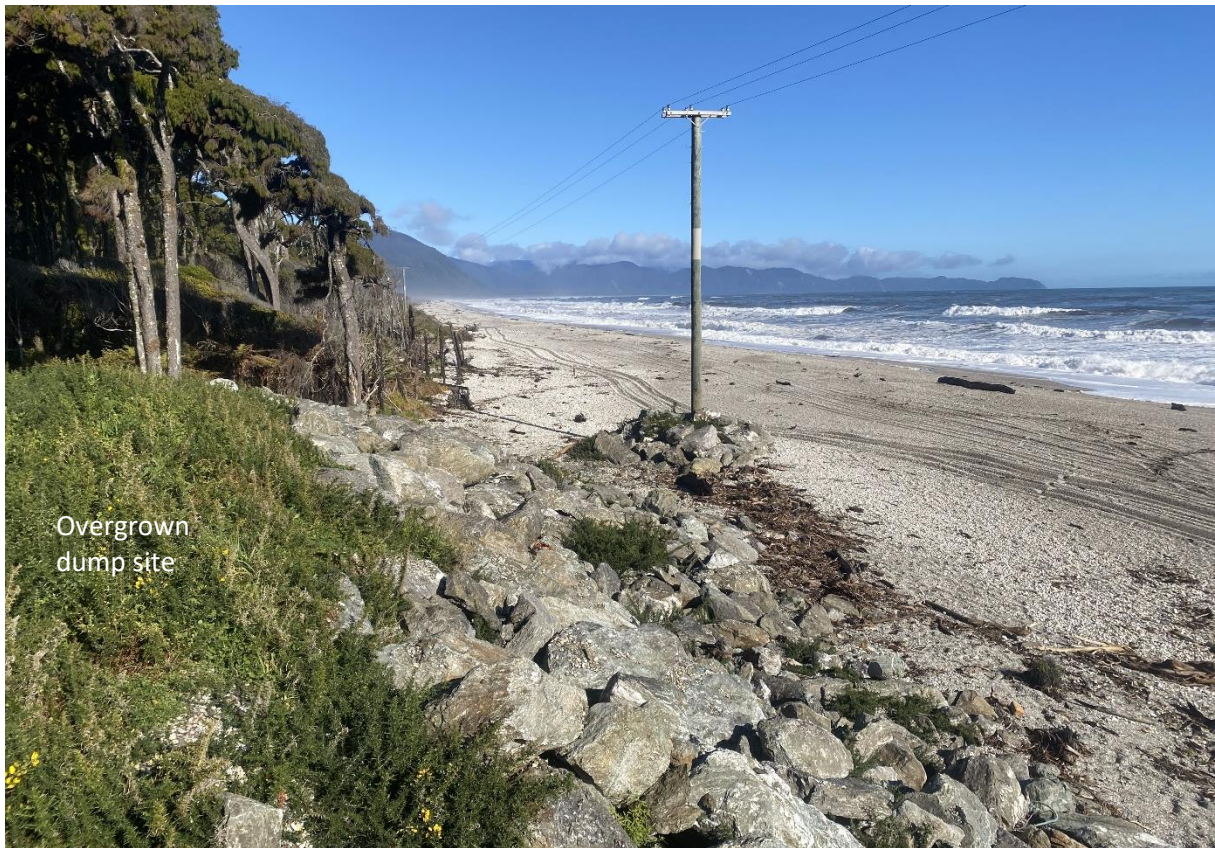
Figure 4-31: Active erosion at old dump site 2 km south of Hannahs Clearing. Erosion has caused vegetation die back, undermined dump (now protected with rock) and exposed the power pole assets. Date 12.8.2021 [Credit: M Allis (NIWA)].
