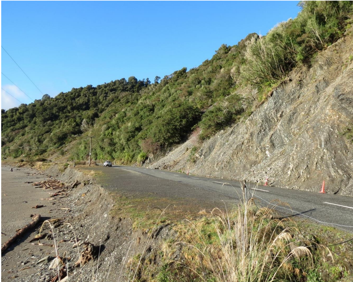
Figure 4-40: Haast-Jackson Bay Road positioned on narrow ledge between landslide prone hillside and beach face. Date 12/8/2021. [Credit: M. Allis (NIWA)].
