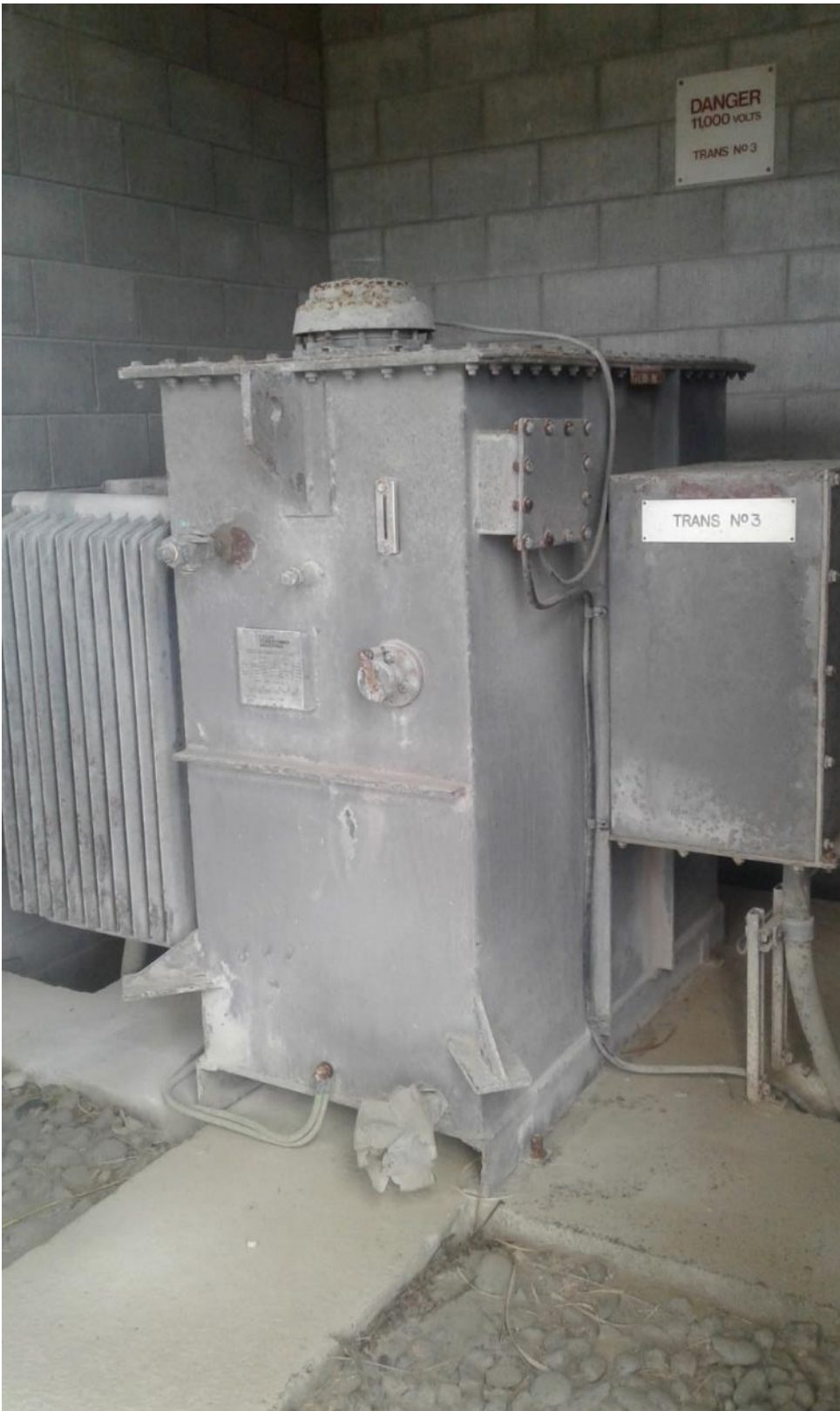
Photograph 22: Crusher – electrical substation transformer.
