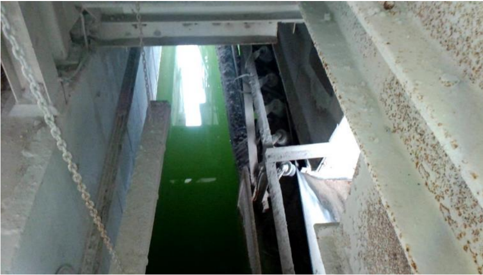
Photograph 23: Crusher – flooded basement.
