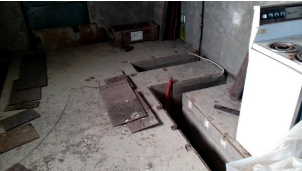
Photograph 15: Electrical substation – internal.
