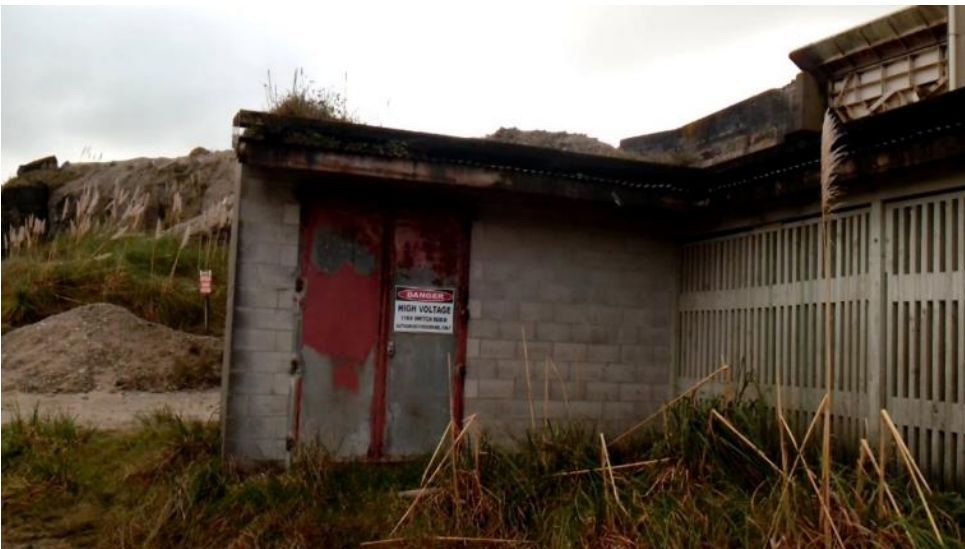
Photograph 21: Crusher electrical substation.
