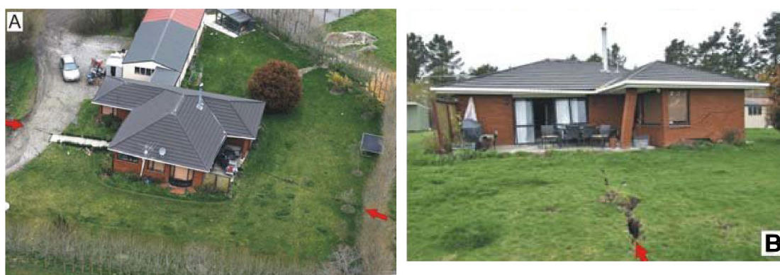
Figure 6.5 Examples of damage to a BIC 2a house caused by surface rupture of the dextral-slip Greendale Fault, near Darfield, during the 2010 Darfield earthquake. Timber-framed, brick-clad house with concrete slab foundation (at most, only lightly reinforced) and light-weight roof that is located within a ~150-m-wide deformation zone accommodating 4–5 m of dextral displacement. The house was badly damaged by distributed deformation and ~0.5 m of discrete strike-slip rupture (red arrows) that enters the house (modified from Van Dissen et al. [2011]).
