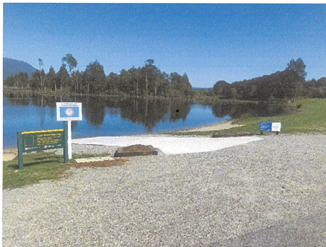
End result, planter boxes now have plants and road marking complete above ramp on new chip seal.
