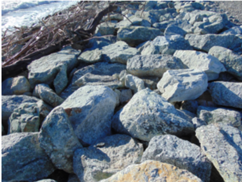
Photo 1 Cobden Armoured |Wall. Simple maintenance for the temporary wall - infill the gaps and hollows. Photo author
