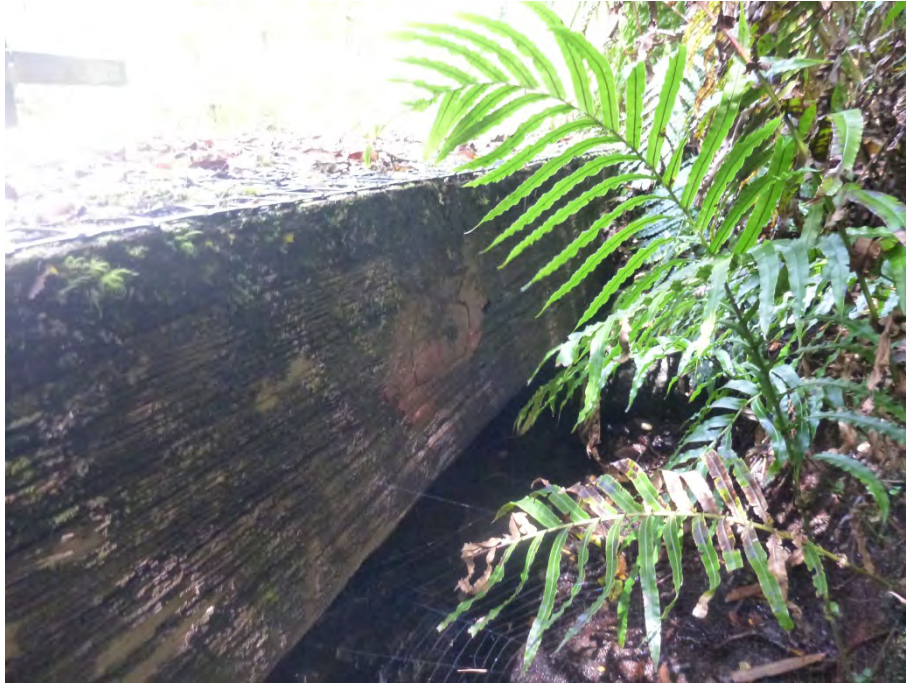
Figure 22. A bridge beam date-stamped 63 (indicating it was installed in 1963, although not necessarily in this location), Footbridge 2.
