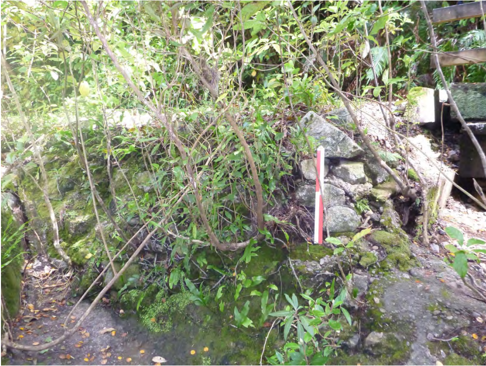
Figure 20. Stone revetting on the corner of the railway formation on the east side of Footbridge 2. Note the concrete in the foreground.
