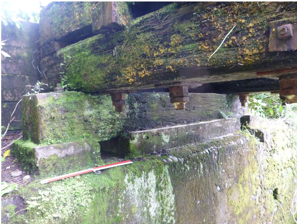
Figure 26. Ballast guard 1 (the modern tanalised timber at rear left) and Pier 1 (the concrete structure in the foreground). Ballast guard 2 and Pier 4 (at the east end of the bridge) were of the same fabric.
