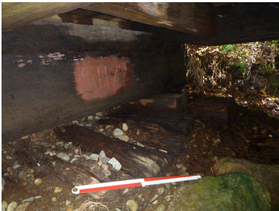
Figure 21. A bridge beam date-stamped SH79, indicating that it was a second hand beam installed in 1979, Footbridge 2. Note also the timber the scale is sitting on. Its function is not clear.
