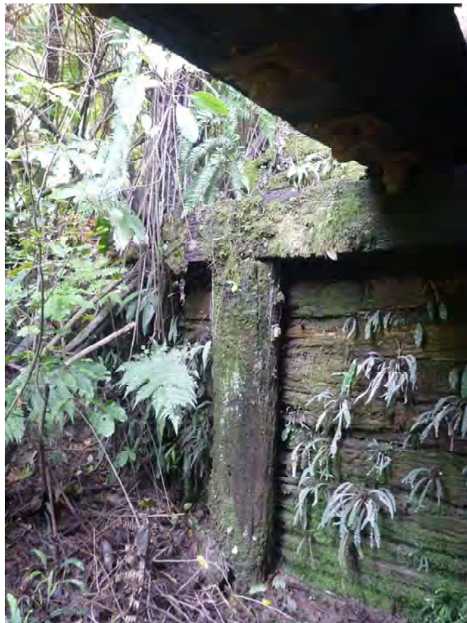
Figure 31. Ballast guard 1 with Pile 1 of Pier 1 in front of it. (Refer to Figure 24 for the numbering system used for the piles – the upstream pile is always Pile 1).
