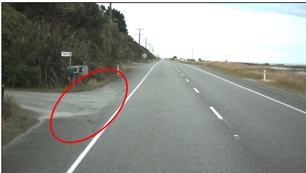
Figure 4: Migration of accessway gravel (circled) on to SH6 on southbound approach to Hokitika (SH6: RP 463 / 4.35; image recorded 7 January 2023. Source: Argonaut, 2023)
