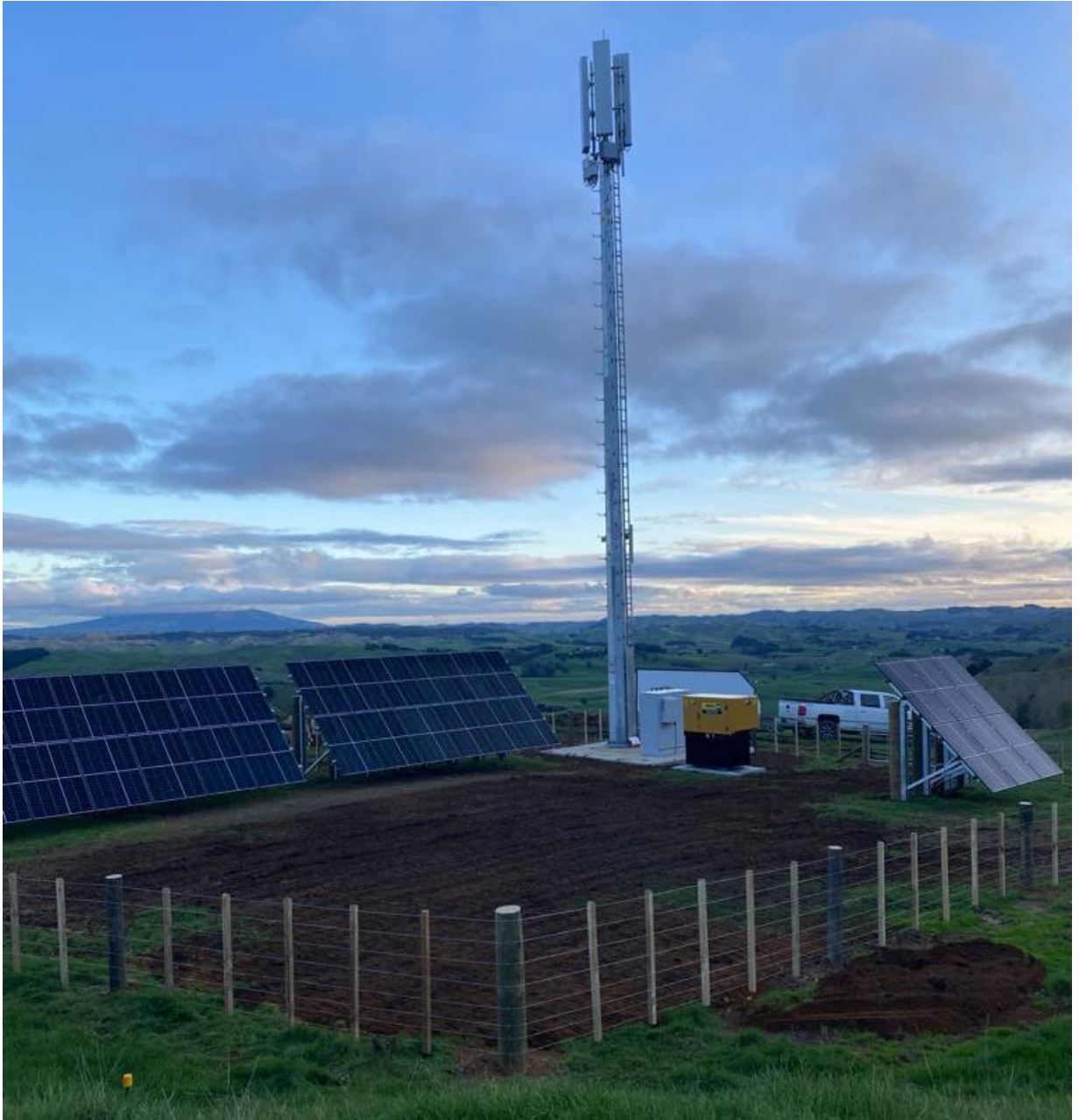
RCG - Te Akau East 20m monopole with diesel generator and solar power
