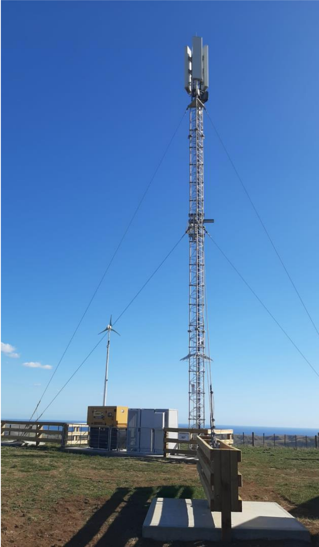
RCG – Waikaretu – 20m with wind and diesel generator
