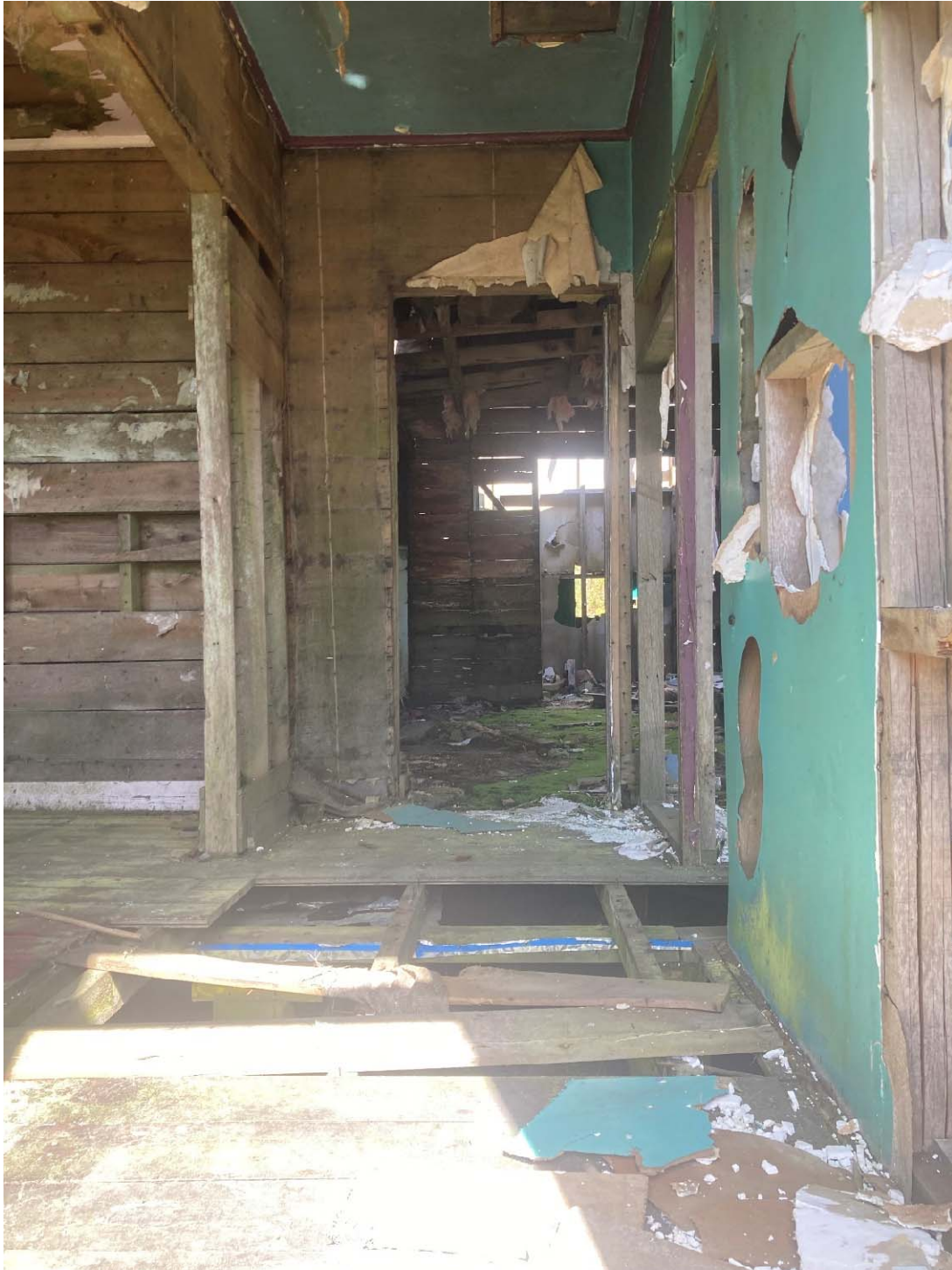
Figure 4: View looking inside of house from front door showing missing floorboards, damage to ceilings, walls, moss growing inside (1 November 2023)
