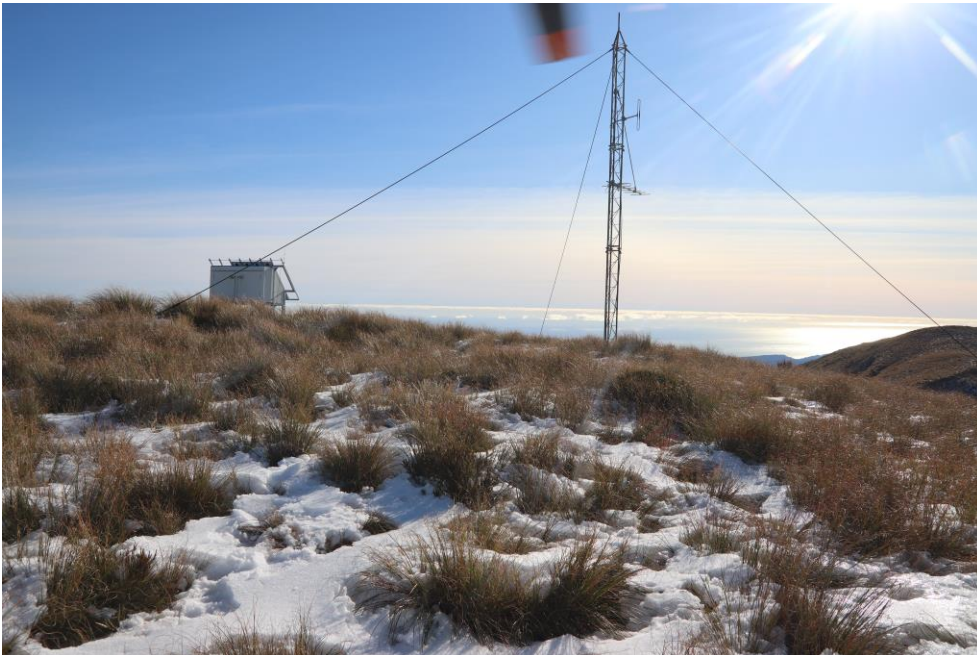
Haast River @ Mt Deelaw repeater tower, with box containing repeater equipment
