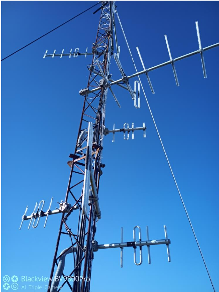
Mt Bonar repeater tower, height is 9-10m
