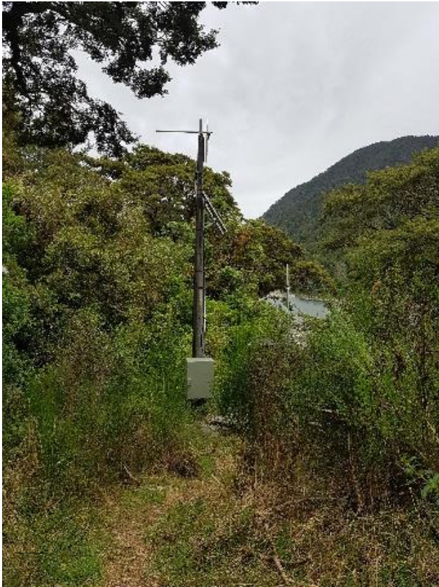
Pole with cabinet, solar panel and antenna, Buller River @ Te Kuha
