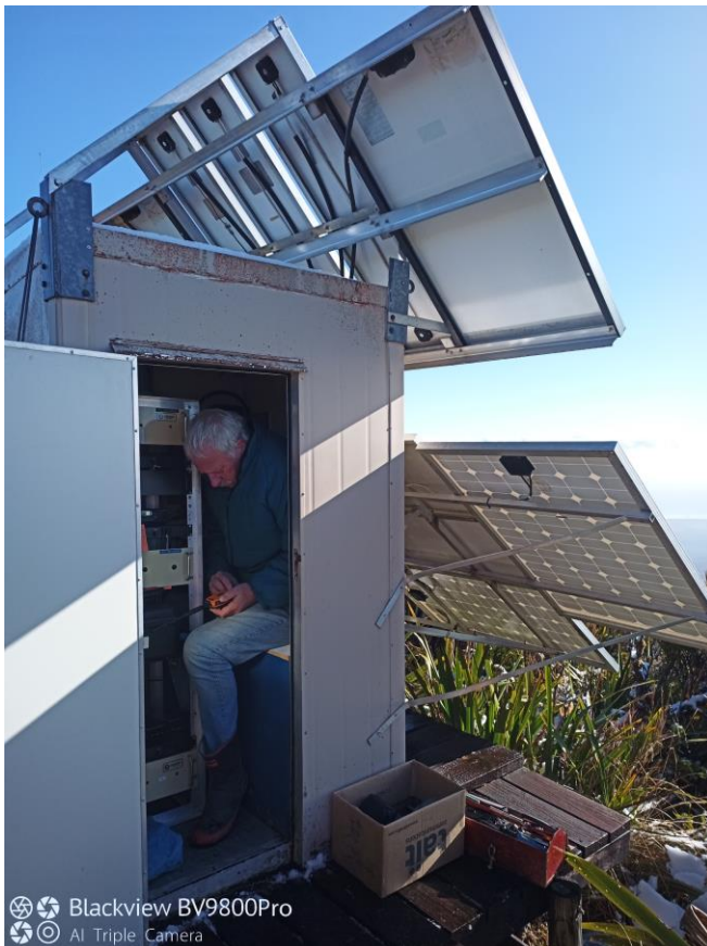
Equipment shed at Mt Bonar repeater site
