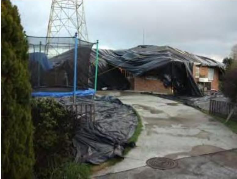
Figure 10 Tower painting in an urban setting, note the extensive polythene sheet protection.
