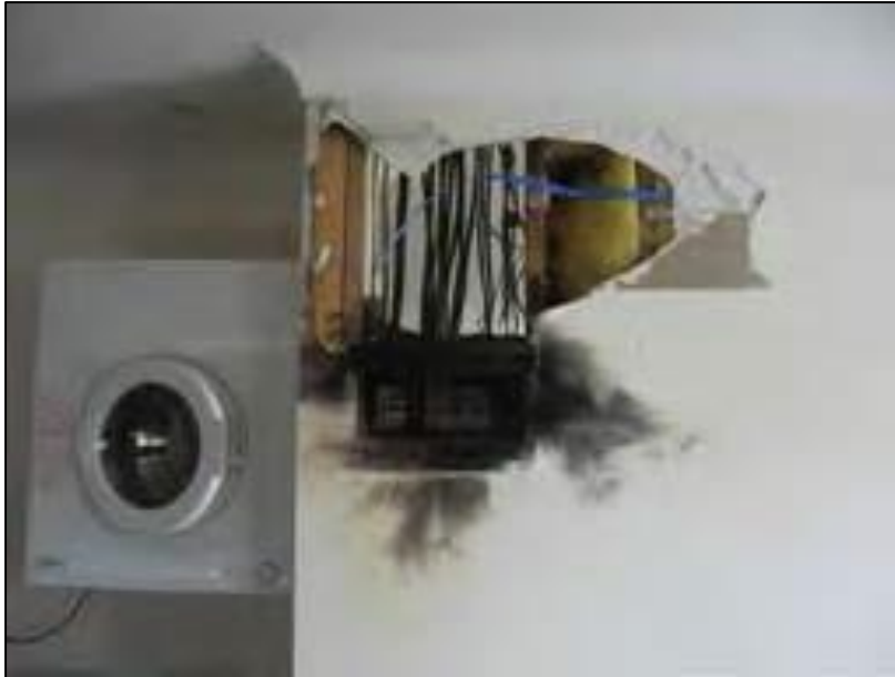
Figure 3 Electrical damage following a conductor drop.
