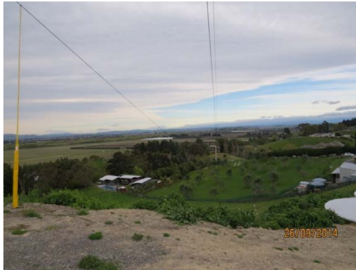
Figure 4. Hastings ground clearance violations
