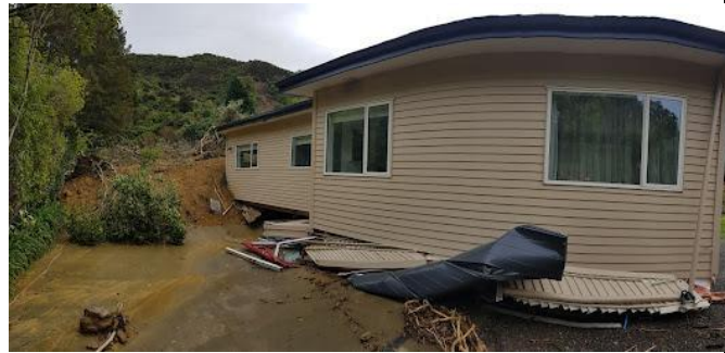
Figure 11. Approximately 2m depth of clay-based landslide debris has pushed this house off its foundation (piles) and moved the building as a complete unit (example from Marlborough).
