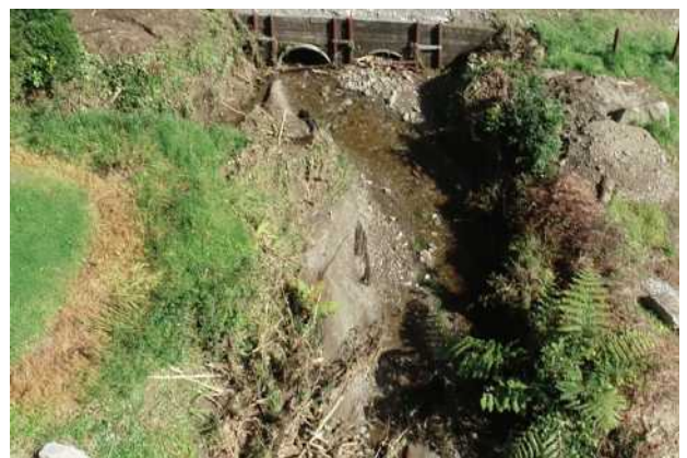
Figure 16. Blocked culverts may have been partly responsible for some of the observed debris inundation in Granity. Photo: BDC.
