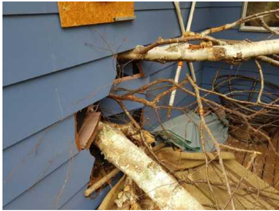
Figure 10. Trees pushed through an external wall of a house impacted by landslide debris (example from Marlborough)
