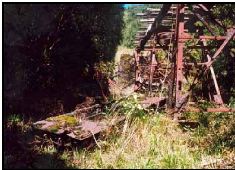
Figure 17 The twisted chassis of a 'Q' wagon underneath the bridge on the upper incline.
