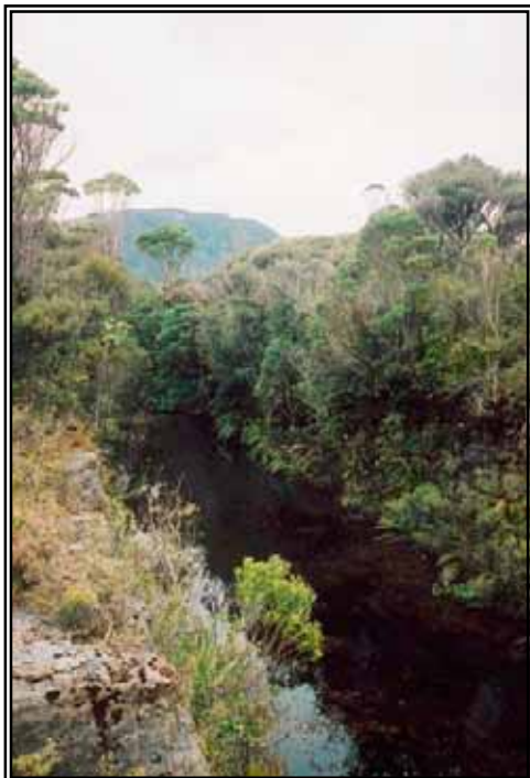
Figure 50 (left) The rope road formation where it passes Denniston. A road embankment has blocked the cutting, causing it to flood.
