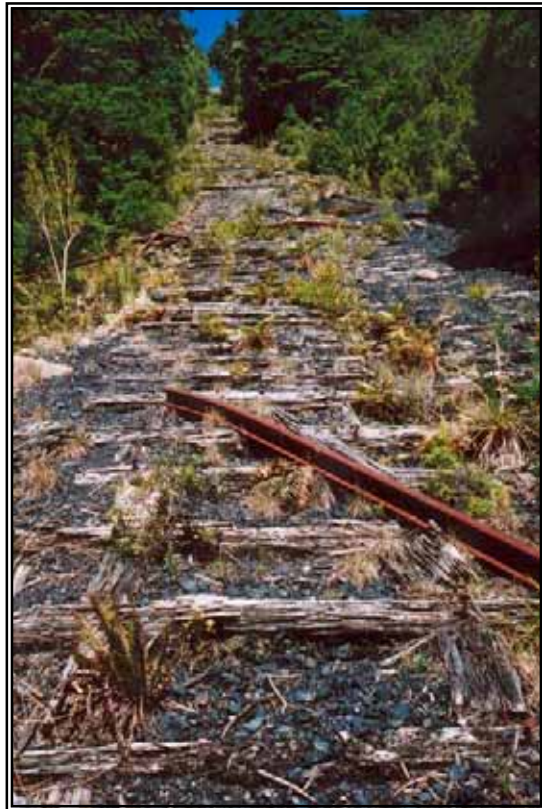
Figure 14 (right) A detail of the upper incline, looking uphill, in 2006. Surviving sleepers and copious quantities of coal are visible.
