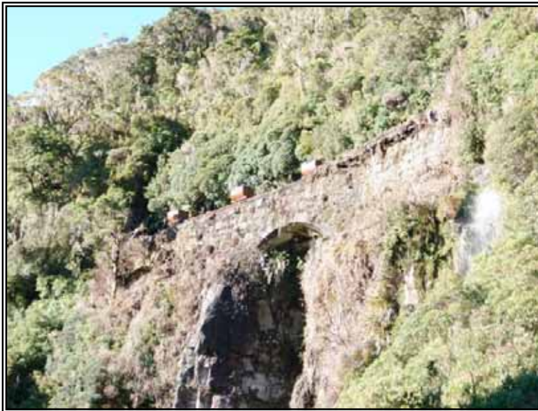
Figure 56 The Banbury Arches in 2007, after vegetation clearance. Note the coal tubs placed on the tramway in the same year (J. Breen, DoC).
