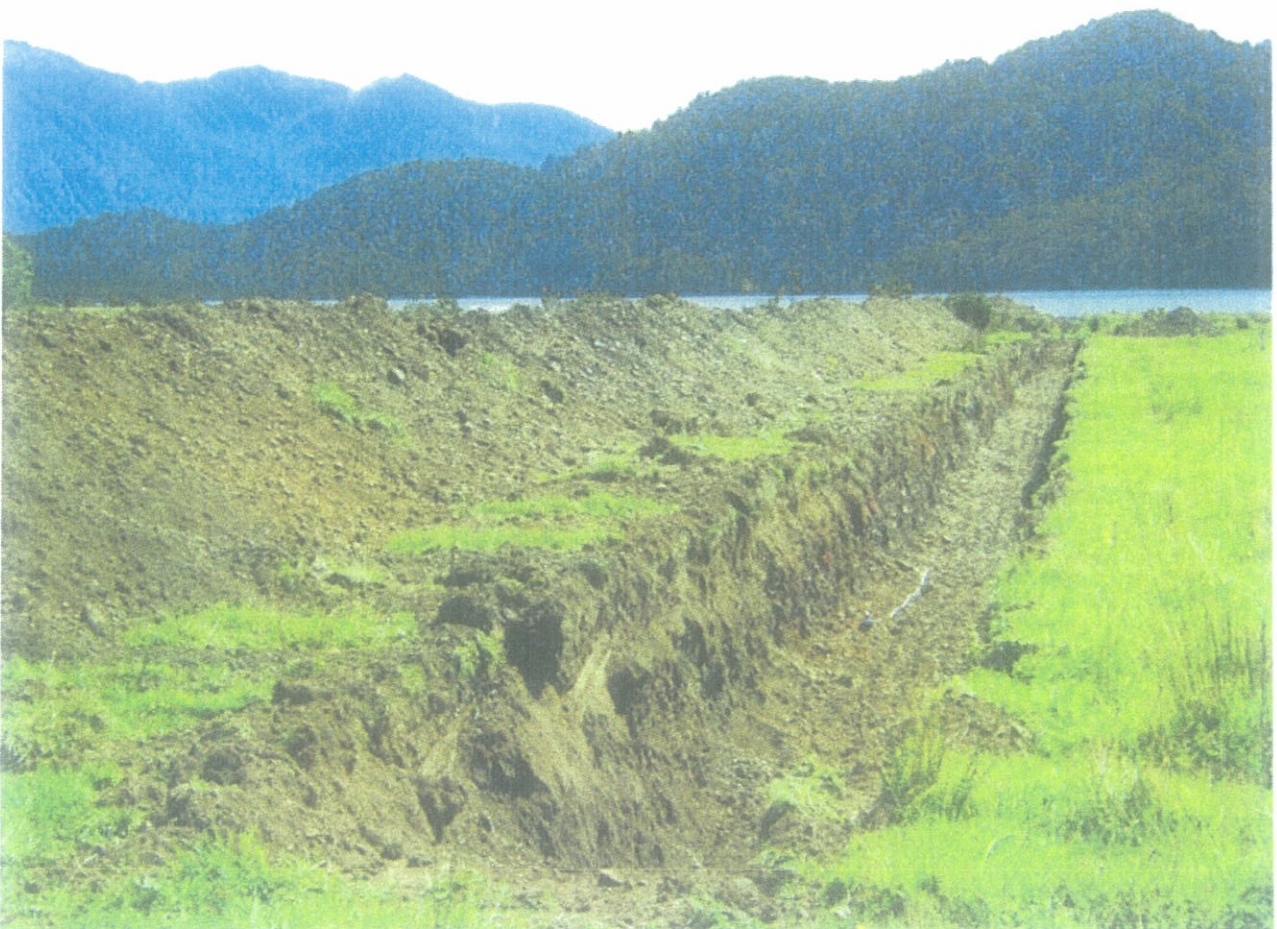
Figure A2: View along Trench C looking north-west towards Lake Poerua, with excavation to typical depth of 2m over distance of ~100m. Note absence of groundwater in trench.
