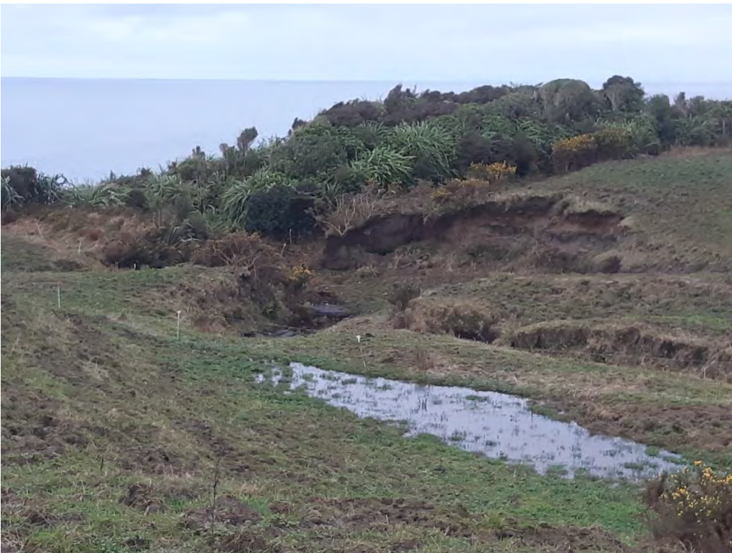
Site Photo 2 Minor slope instability associated cut slope along an access ramp to a creek crossing
