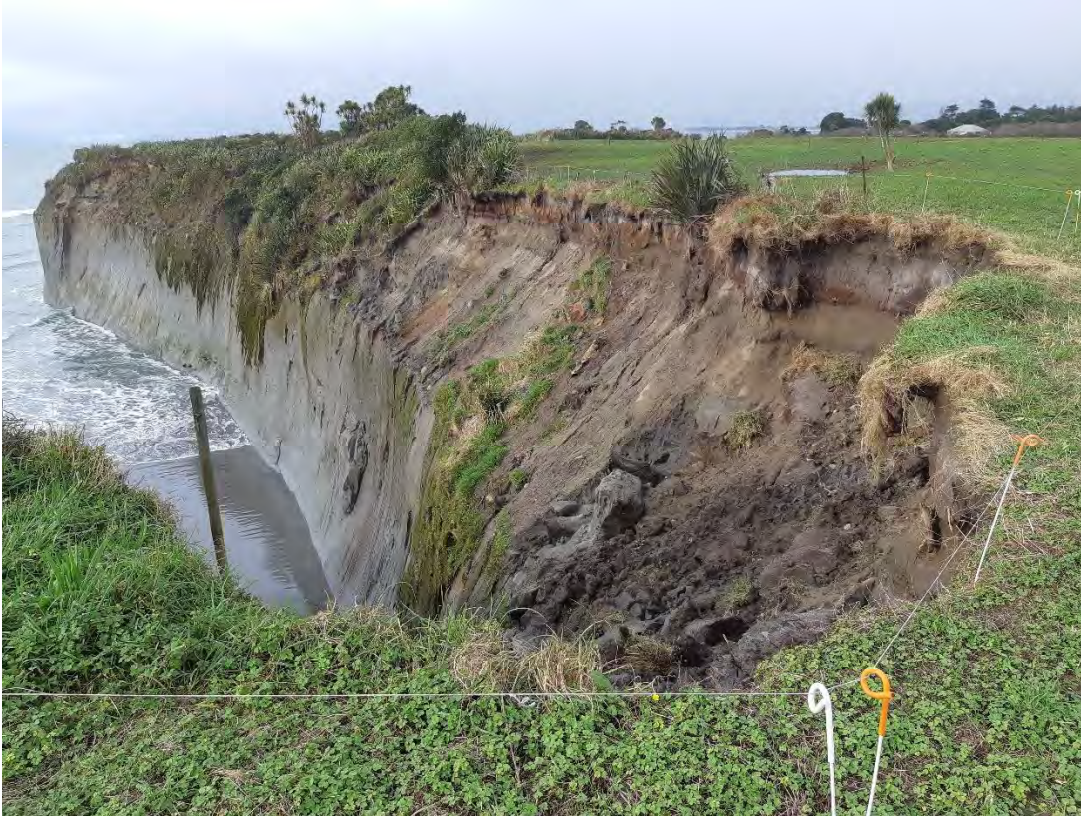
Site Photo 8 Recent failure in Quaternary unconsolidated sands along the crest of the Omau Cliffs. Lack of extensive iron cementation makes this section more prone slope failures
