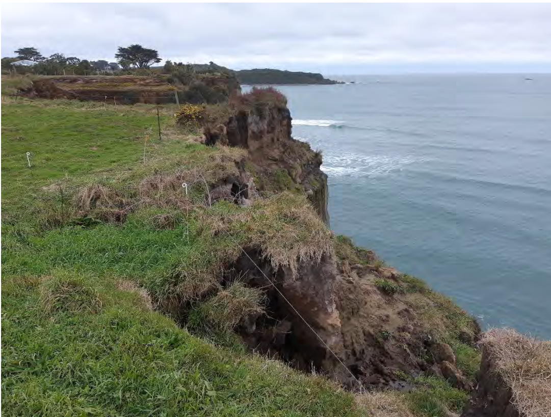
Site Photo 9 Recent slope failure along the cliff crest caused by water intrusion from natural drainage of the terrace. West end of the subdivision. Lack of extensive iron cementation makes this section more prone slope failures
