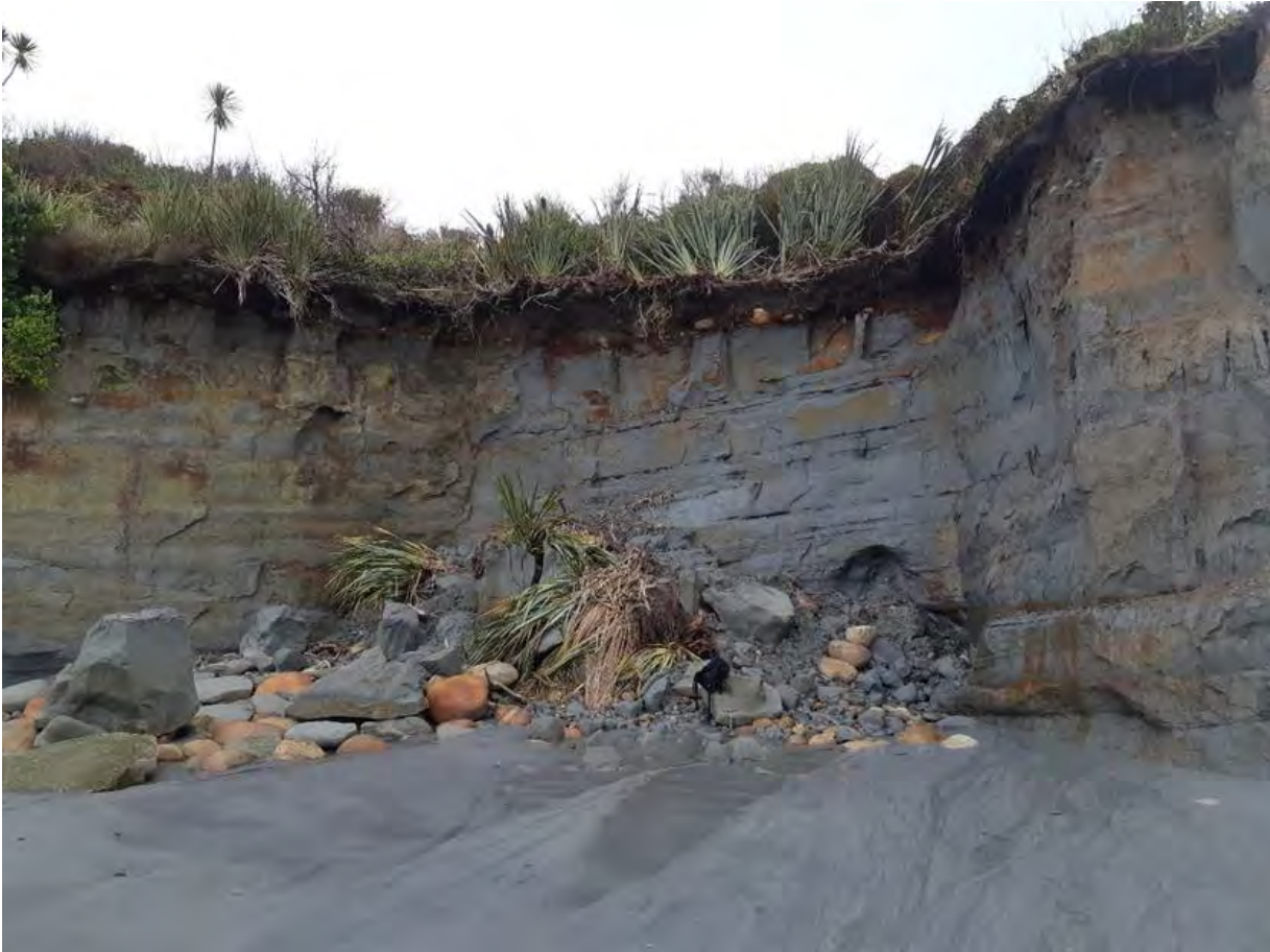
Site photo 4 Recent significant failure likely due to undercutting of the toe by wave action causing collapse of the overhanging rockmass. Daypack in the centre of the photo for scale. Note the typical step planar failure plane behind the spoil indicating
