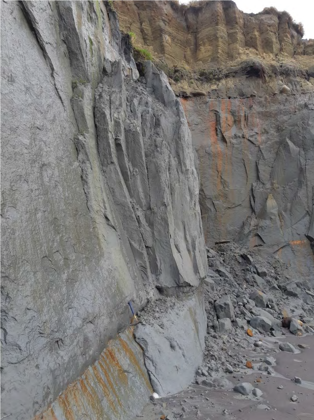
Site photo 3 Typical slab failure along SW-NE and WNW-ESE orientated, very steeply inclined to subvertical, planar, moderately widely spaced (0.2-0.6m) persistent joints observed in the mudstone along the beach below Omau Cliffs. The intact strength of the mudstone ranges from extremely weak to weak .
